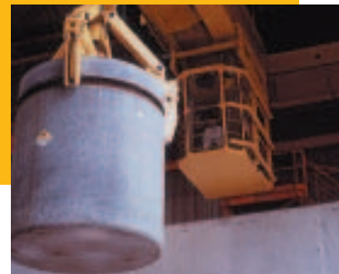
Lowering a concrete shell into a repository structure (the Aube LILW disposal facility)
