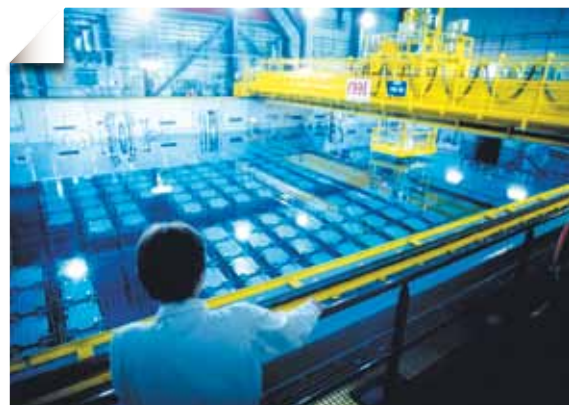
Storage of spent fuel in fuel cooling pool
