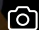
Deconstruction worksite of the Chooz A nuclear power plant: deconstruction of the cavern
